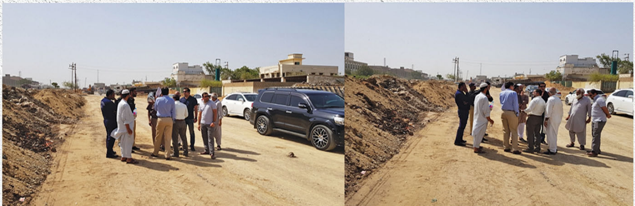
PTA (S.Z) Infrastructure Committee Members led by Chairman, Mr. Aziz Ahmed visited the site of GC-Bin on Road-5000 for its expansion & rehabilitation work to be done on 27-03-2018.
