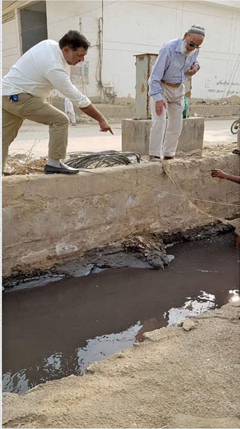
MR. SHEIKH MUHAMMAD IMRAN, VICE CHAIRMAN PTA (S.Z) BRIEFING CONSULTANT ABOUT ONGOING INFRA-STRUCTURE PROJECTS IN SECTOR 7/A, KIA.
