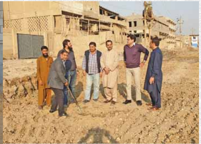
Ground Breaking Ceremony Of Construction Of Southern Avenue Road In Sector 7-A.
